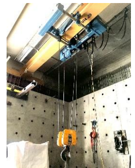
10 ton overhead crane at More Hall
