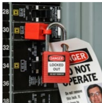
Circuit breaker lockout device locked and tagged out
