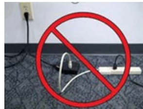
Surge suppressor daisy-chained to an extension cord, not allowed.
